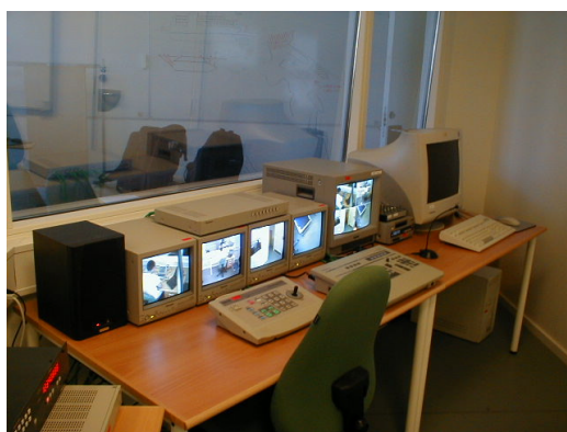
Figure 4. Control room: equipment for operating the motorized video cameras in the subject room.
